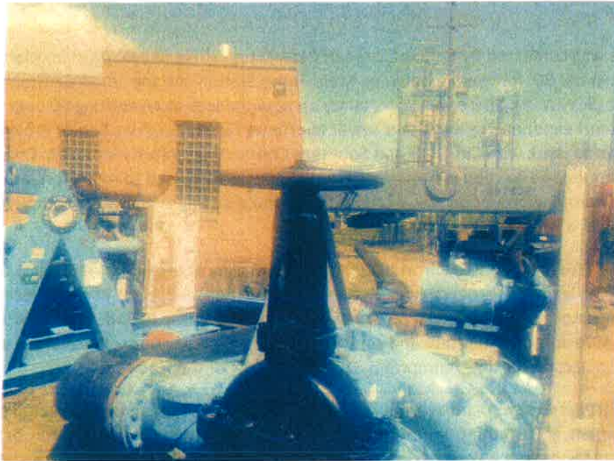
TEMPORARY BYPASS PUMPS AND FORCE MAIN TO SCWWTP
