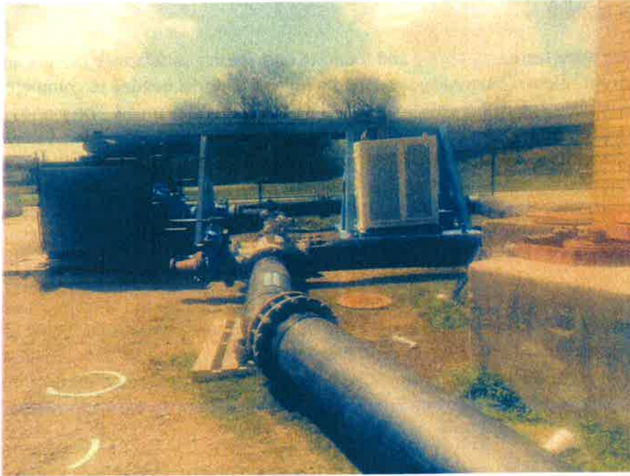
TEMPORARY BYPASS PUMPS WITH SUCTION MANIFOLD AND DISCHARGE FORCE MAIN
